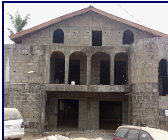
The St. Paul congregation were recently able to complete the metal roof on their new church.
